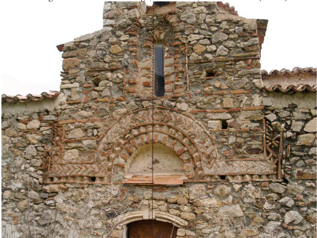
Fig. 23. Detail of the south façade of the church of St. George, Bosinianika (author).
