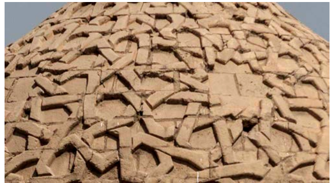
Figure 21: Complex of al-Ashraf Barsbay, detail of courtyard dome chamber (photo: B. O’Kane).
