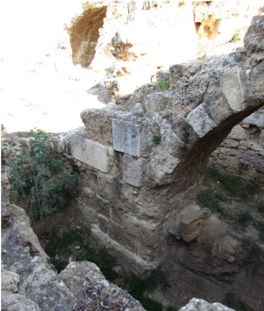
Fig. 3: Grand Baths at Salamis-Constantia. Internal flying buttresses near the praefurnium. Substructure is beneath floor level.
