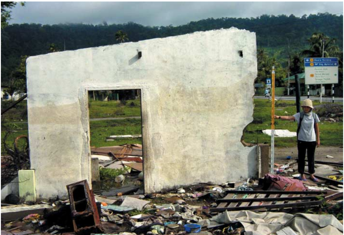
Plate 2 Looking north at a watermark recorded as 383 cm (elevation of water above MSL), 160 cm (water depth) in Figure 2, in the zone of maximum damage between Kuala Teriang and Kuala Melaka. This is the only wall of this brick house that was left standing. The wall is oriented perpendicular to the flow, which was from left to right. A brown watermark slopes irregularly upward from 140 cm above the ground to the left (marked by an arrow), to 180 cm to the right. The main road through the Kampong is visible in the background
